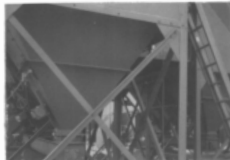
2P-200 on Dust Collector Hoppers
